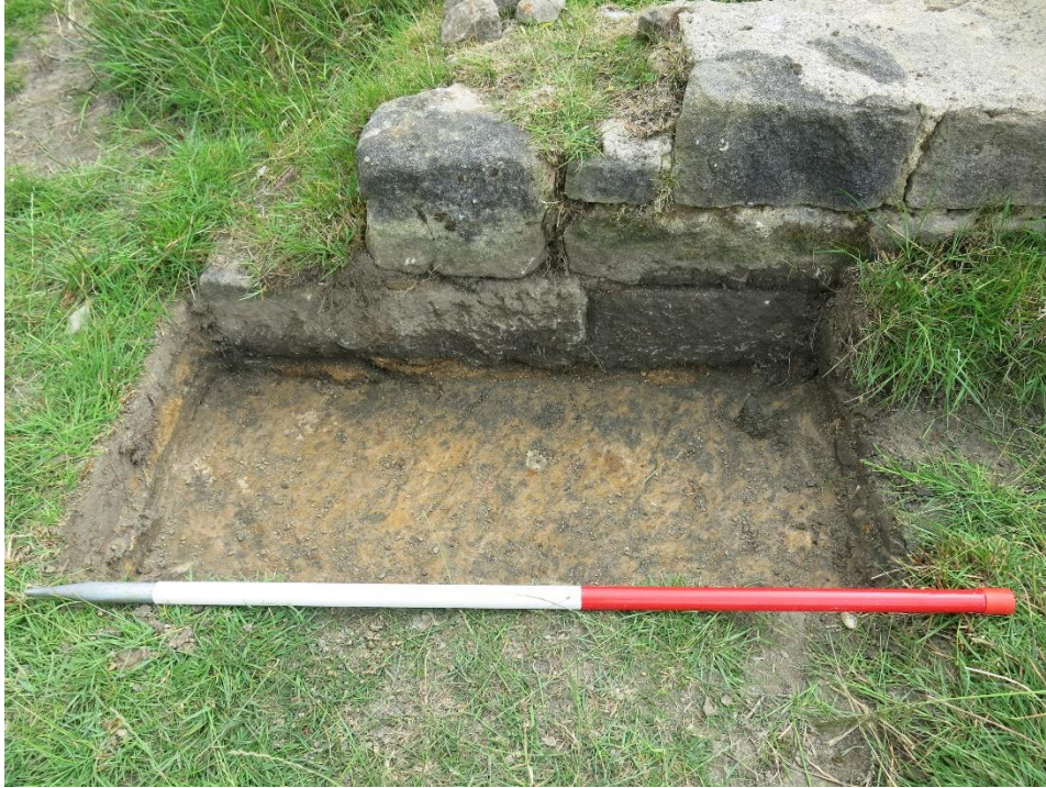
The photo shows the well-dressed base stones sitting on a bed of dark yellow mortar.
